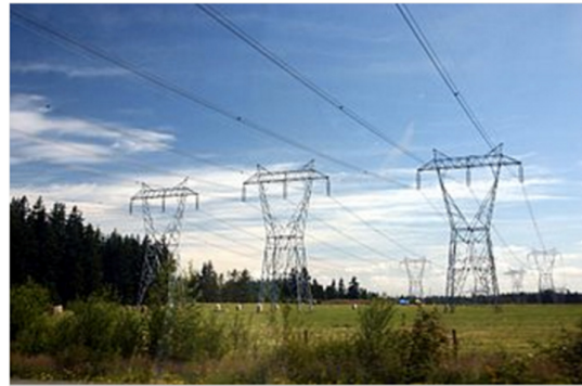
Three-phase electric power transmission lines
